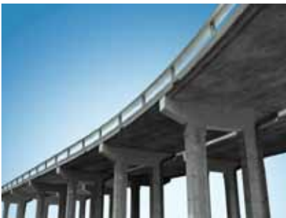
A concrete highway bridge: has it been made well enough to last?
