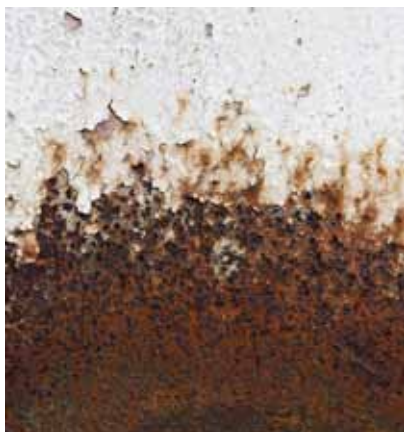
Rust forming on painted steel
